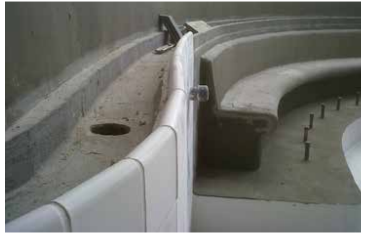
Sistema S9 Wiesbaden / Acquaworld / Concorezzo, Italy
